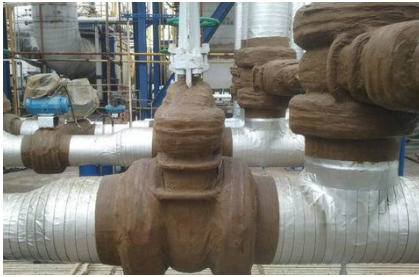
Valves, flanges and fittings
