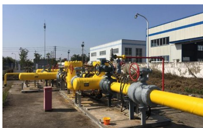
Gas distribution main
