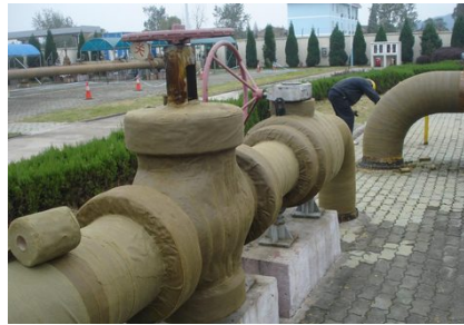
Local corrosion at fittings
