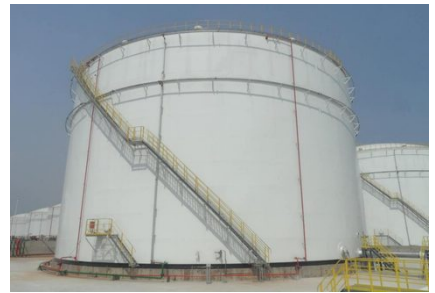
Above-ground storage tank
