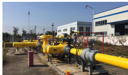
Buried and above-ground pipework
