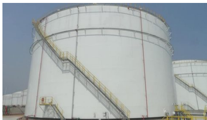
Storage tank base
