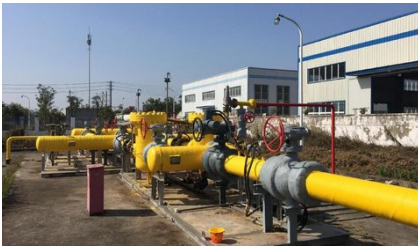
Gas distribution main
