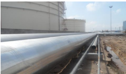
Buried steel pipeline
