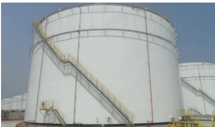
Storage tank shell
