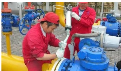
Buried valve assembly
