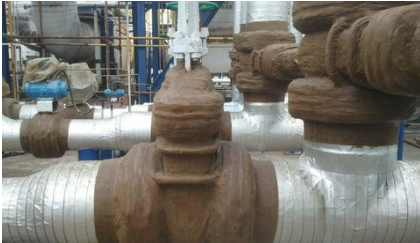
Valves and fittings
