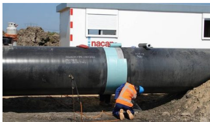
Buried pipeline field joint
